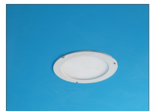
Internal recessed lights
