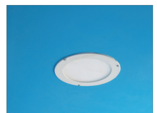
Internal recessed lights
