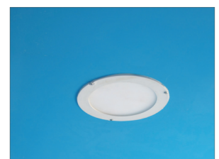
Internal recessed lights
